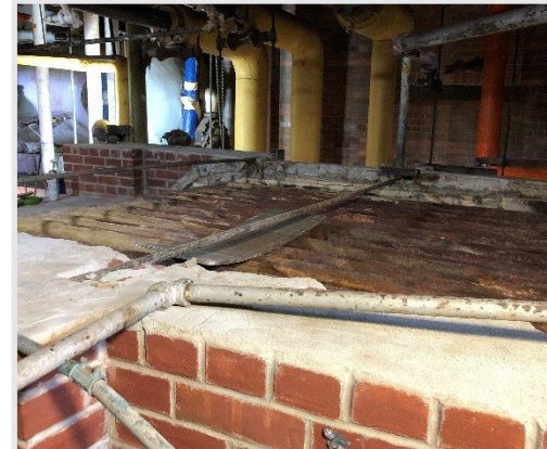
After Photo - Top of Boiler
