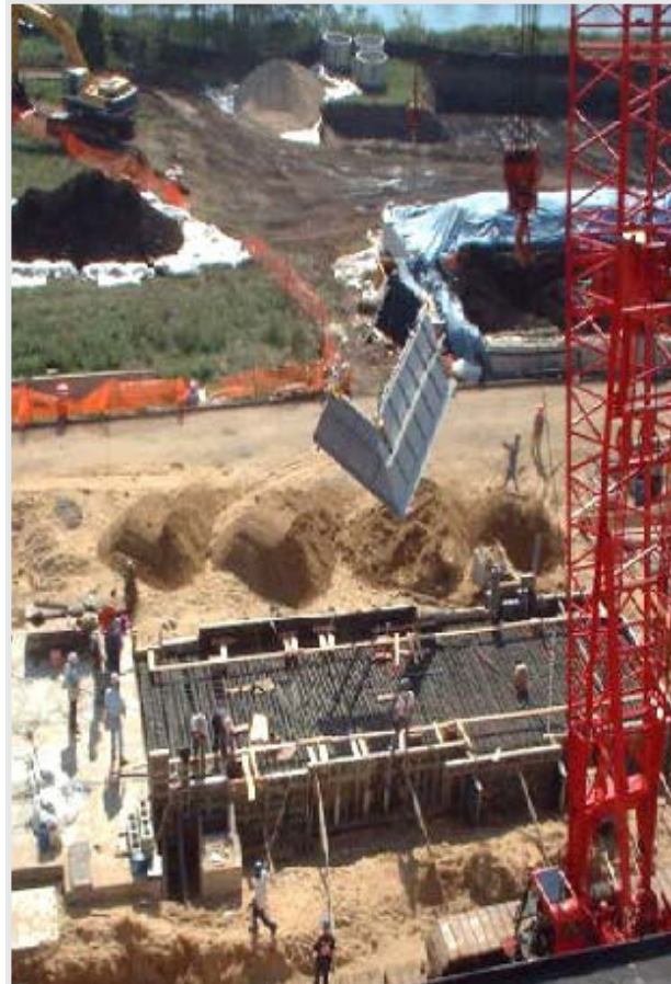
Freeport Electrical Power Plant 2, Freeport, NY
