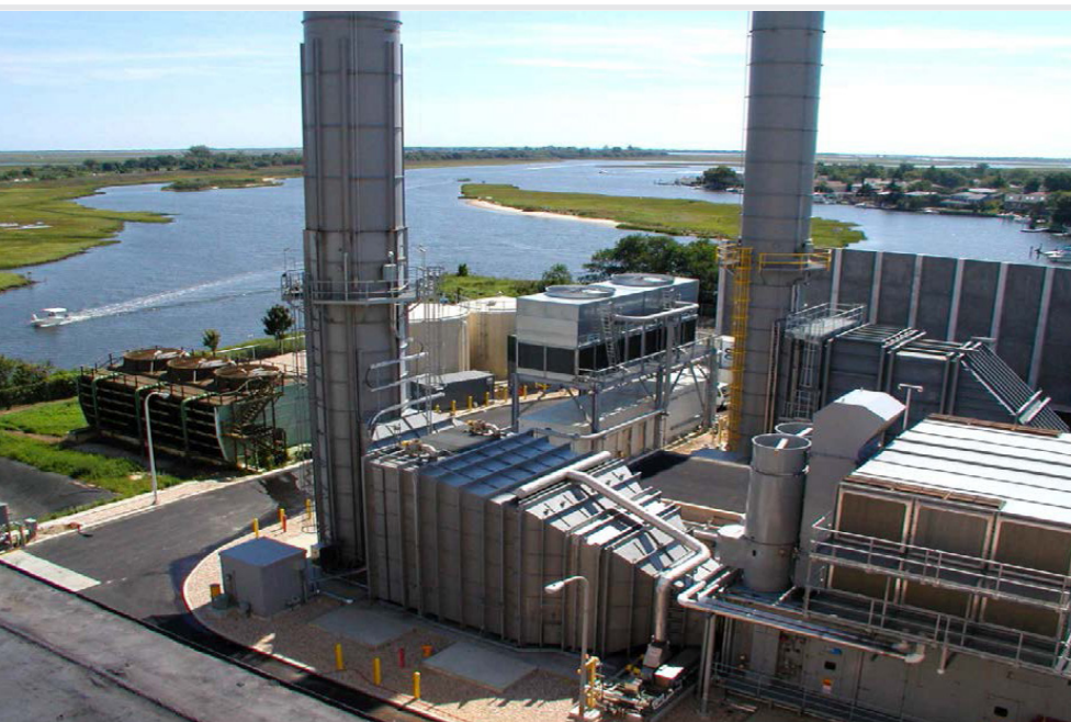
Freeport Electrical Power Plant 2, Freeport, NY
